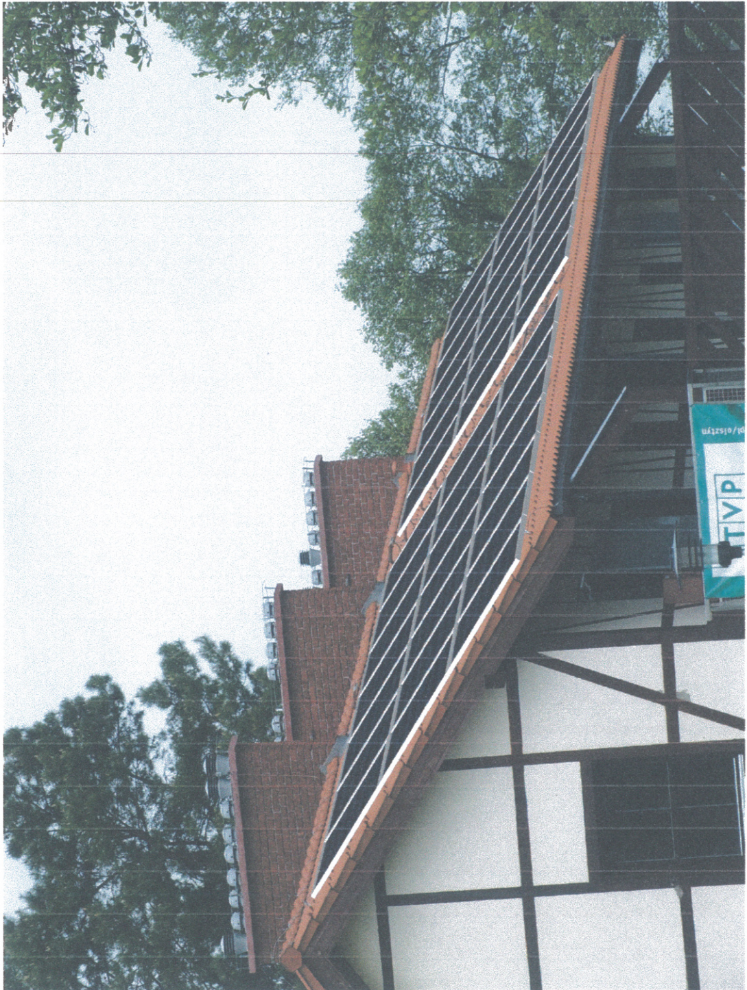
42 panele PV po 270 Wp
